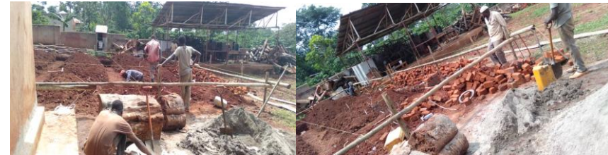
Day one and the trenches for the footings are going in, is that the foreman I see 😊
